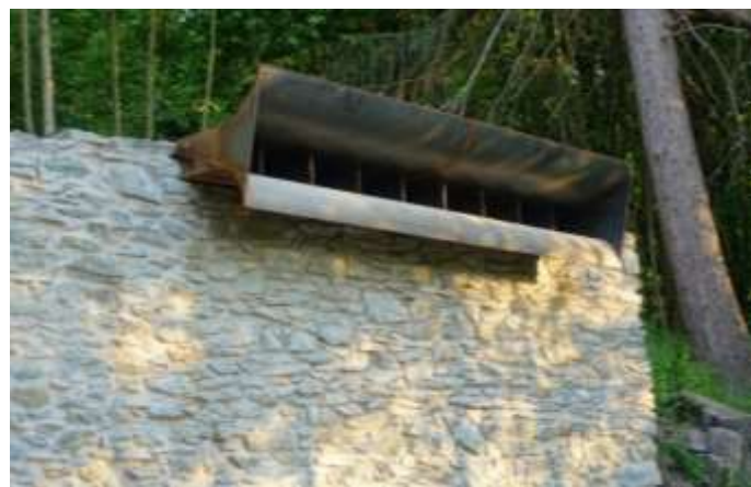
Fig. An object with a "mouth-like" steel structure was installed to prevent predators from catching bats in the FFH site (Flora-Fauna Habitat) at Büchenberg (Saxony-Anhalt, Germany).
